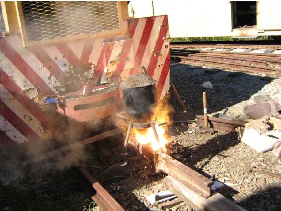
The first Thermit weld being used to extend the siding in front of the BLC.
