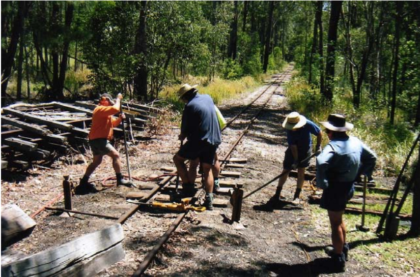
Renewal of defective sleepers is an important activity to maintain the integrity of the mainline. On 13 th October 2007, sleeper renewal was in progress near Storybrook.
