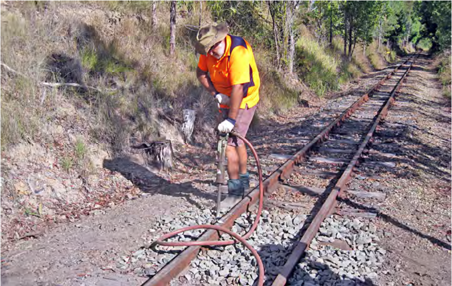
Greg Stephenson packing steel sleepers installed at track joint, 2014. Terry Olsson photographer.
